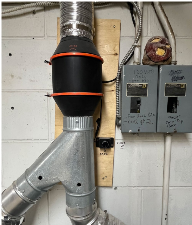
New motors in the kiln room, Fall 2024.
